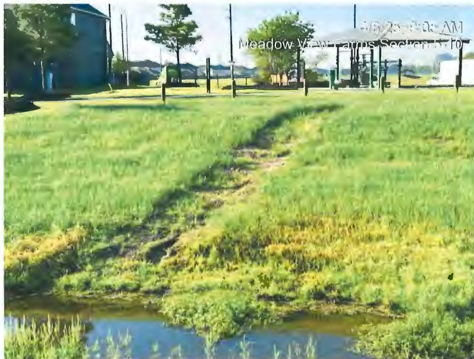
Drain line with erosion
