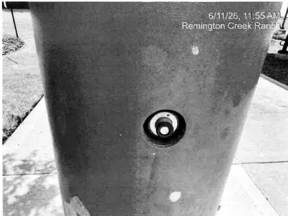
Remington Creek Ranch Exercise Park – broken water fountain, water off at meter
