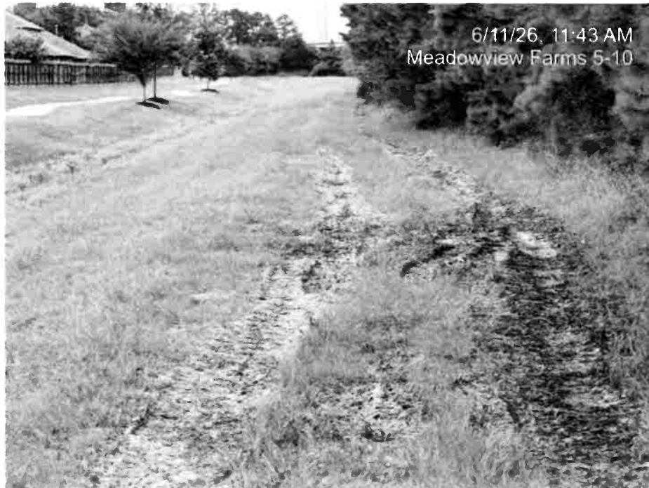
Meadow View Farms Sections 5-10 – Ruts along top of pond
