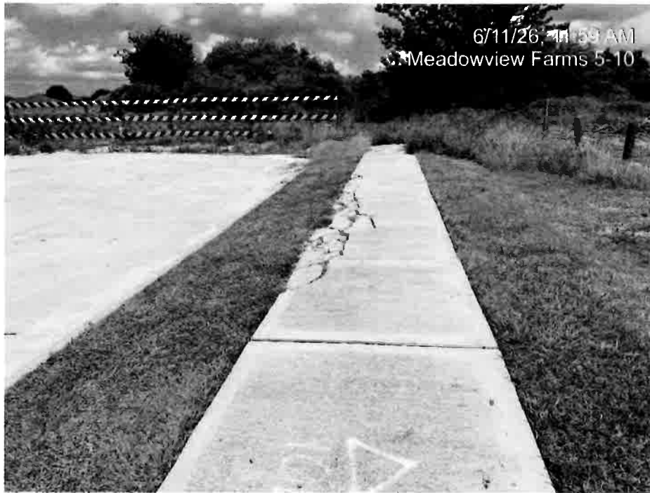
Remington Creek Ranch Exercise Park – damaged sidewalk near dead end
