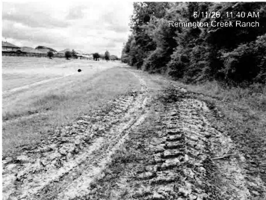
Remington Creek Ranch – Ruts along top of pond Richey Road access
