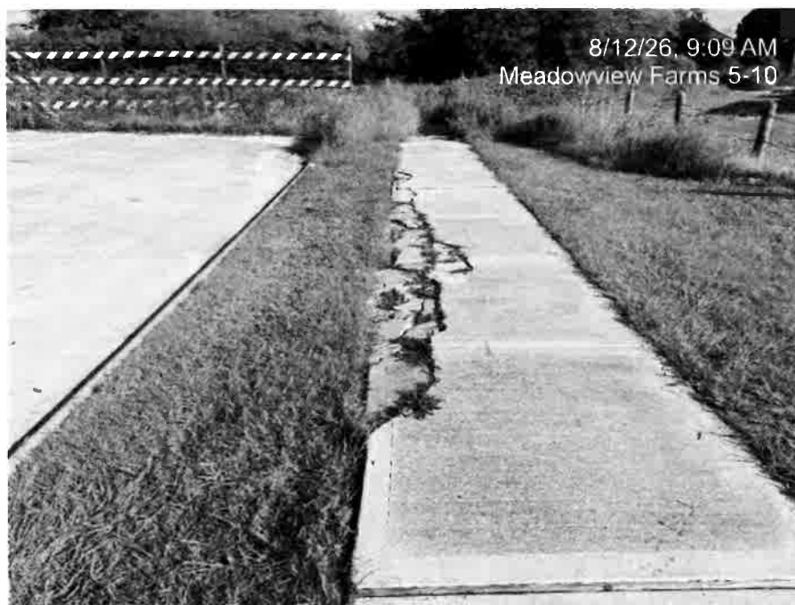
Remington Creek Ranch Exercise Park – damaged sidewalk near dead end
