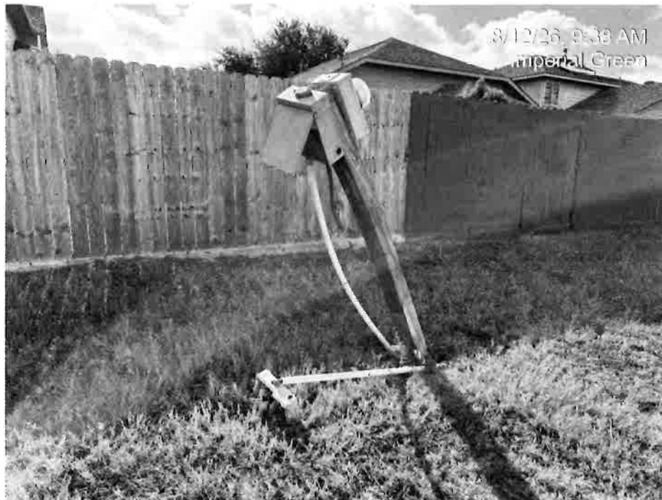
Imperial Green – broken sprinkler box/post
