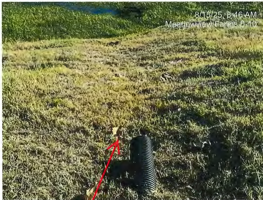
Drain line with erosion
