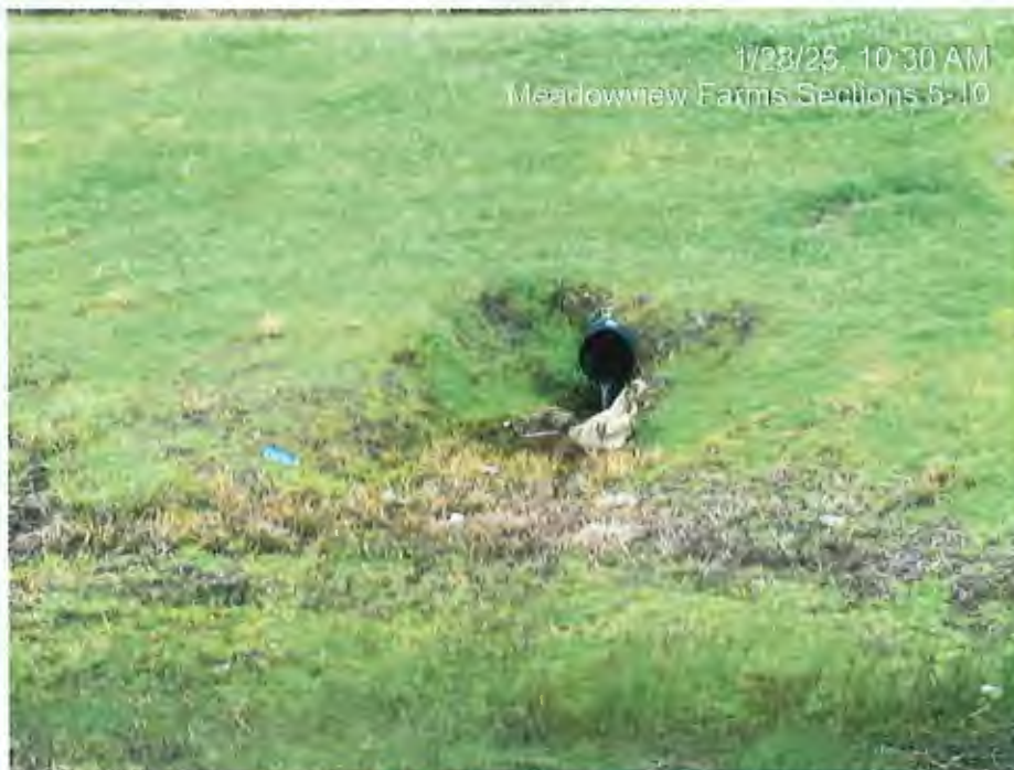
Drainage pipe doesn't extend to the toe of the pond, East side of pond
