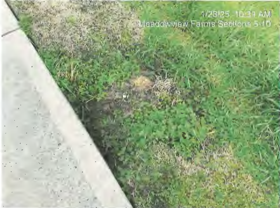
Void around sidewalk, West side of pond
