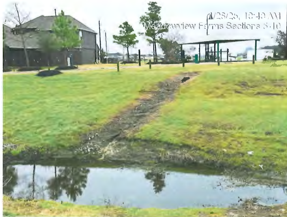
Drain line with erosion
