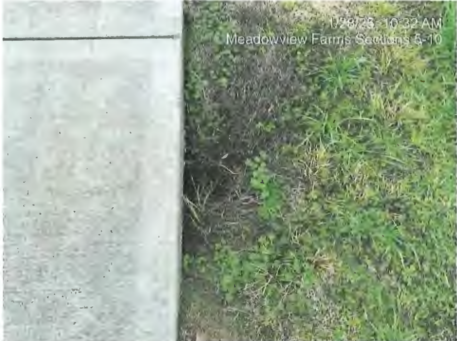
Void around sidewalk, West side of pond
