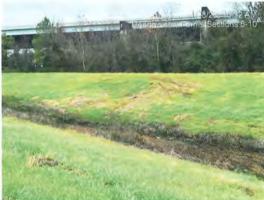
Washed out area near the Northeast corner of the pond
